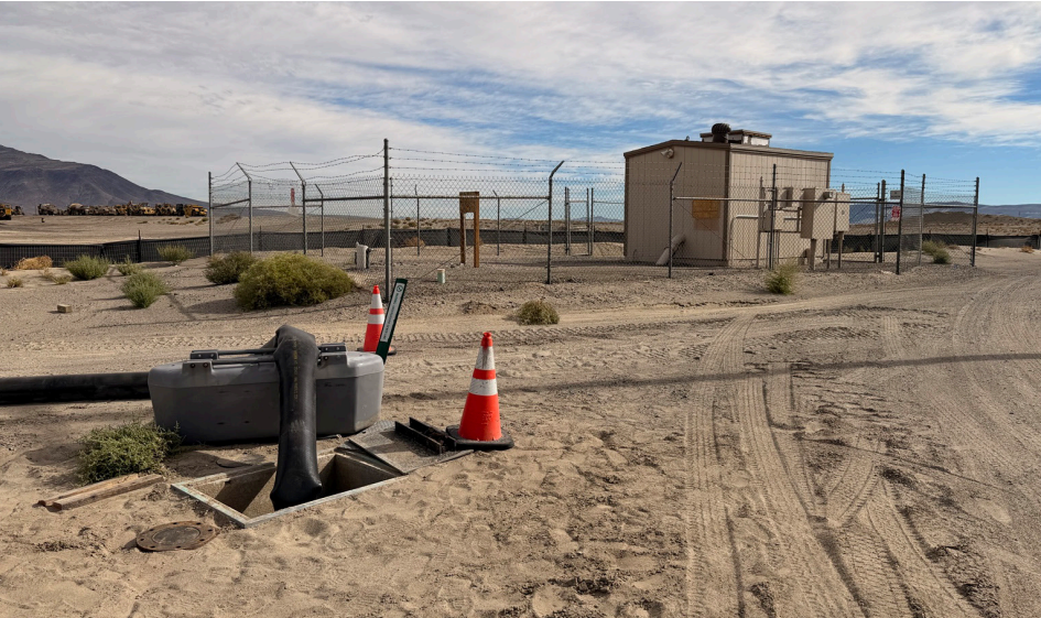
The City of Fernley installed a bypass around the lift station that failed on Friday, Sept. 11. In the background is Well 9 that provides municipal water to the City of Fernley. The city has said that the well was not affected, but in an abundance of caution, will be monitored and sampled.
