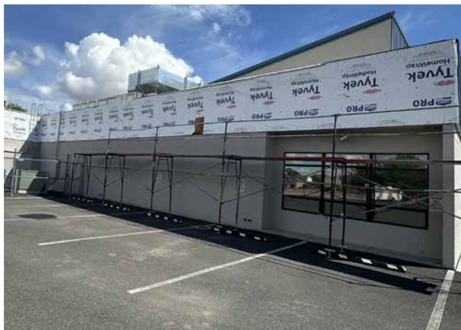
The reopening of the Fernley Swimming Pool is being delayed several weeks because of an issue with the production and delivery of materials for the new roof. Photo by Robert Perea
