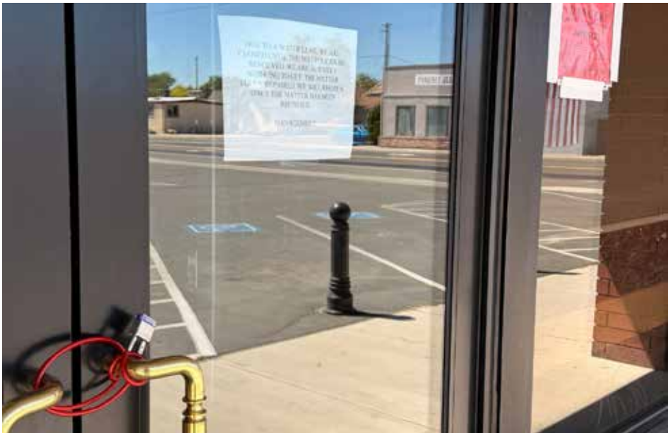
The state department of health and the City of Fernley shut down the Wigwam last week because of water damage in the restaurant ceiling .Photo by Rachel Dahl.
